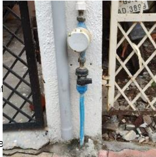
24X7 Water supply and Metering
